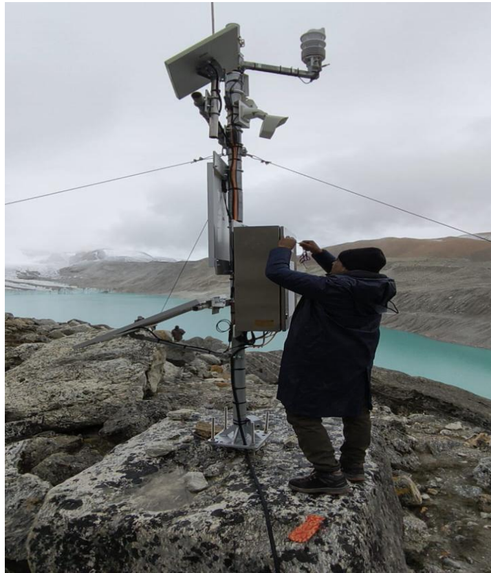
Figure 8: AWS installed at South Lhonak Lake on Right Moraine
