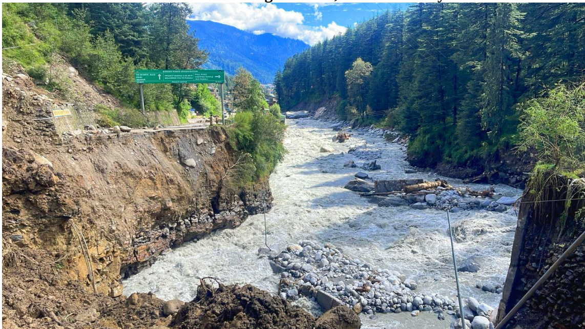
NH damaged in Disrict Kullu
