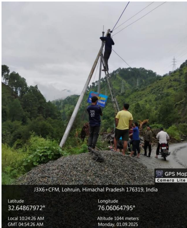
Electricity Supply being restored by HPSEBL
