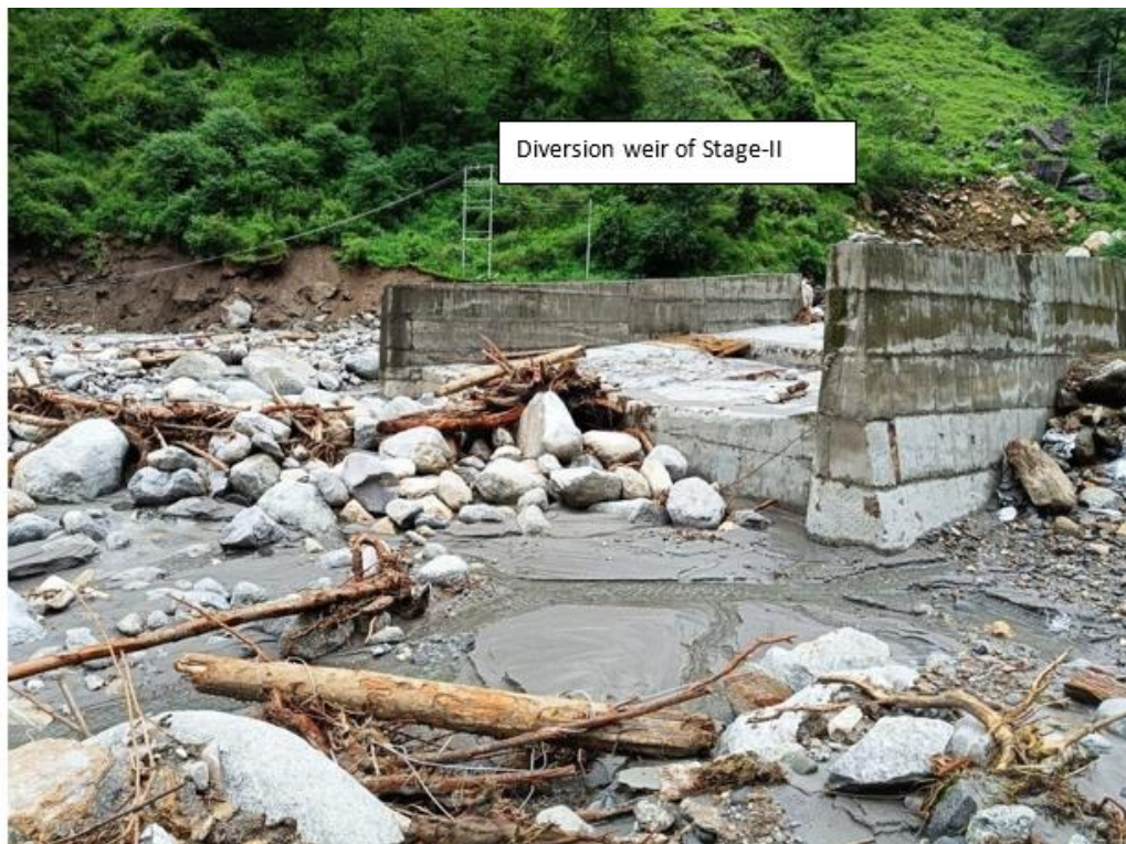
Figure 4 Damaged Diversion weir of Ganvi HEP-II
