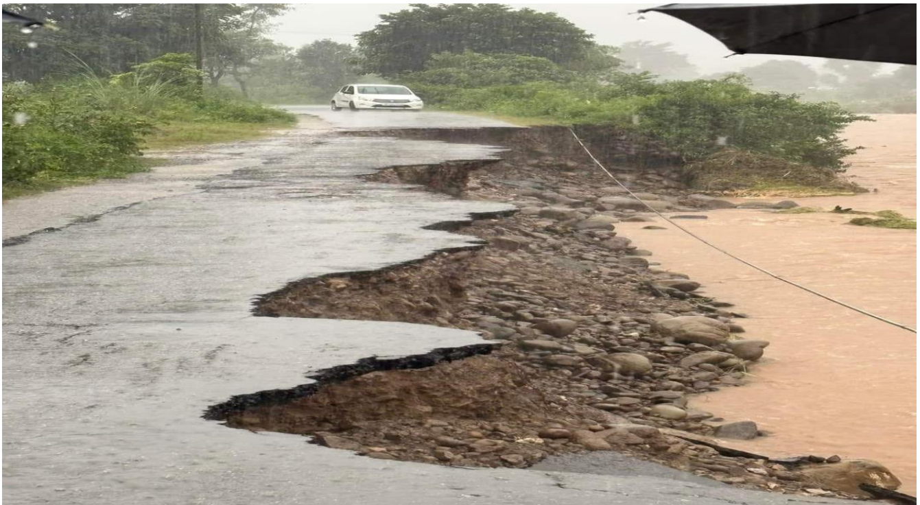
Damages at Sub-Division Paonta Sahib, district Sirmaur
