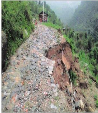
The damaged Neul-Shanshar road in Sainj valley of Kullu.
