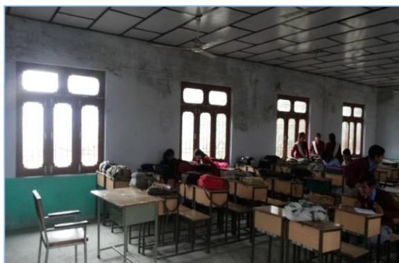
Fig. 1 Poor design-wall length > 8m ( GSSSI Nalti)
