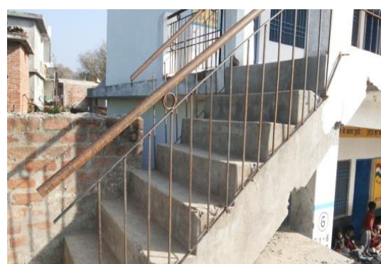
Fig.28 Improper finishing of handrail (GSSS Tal)
