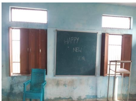
Fig.23 Wrong placement of greenboard causing glare.(GHS Bralhari)
