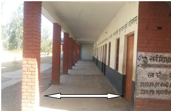
Fig.21 Corridor area limit exceeded (GSSS Bhota)
