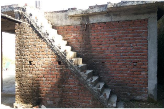
Fig.25 Open stairs not as per standards (GPS Pananyala)
