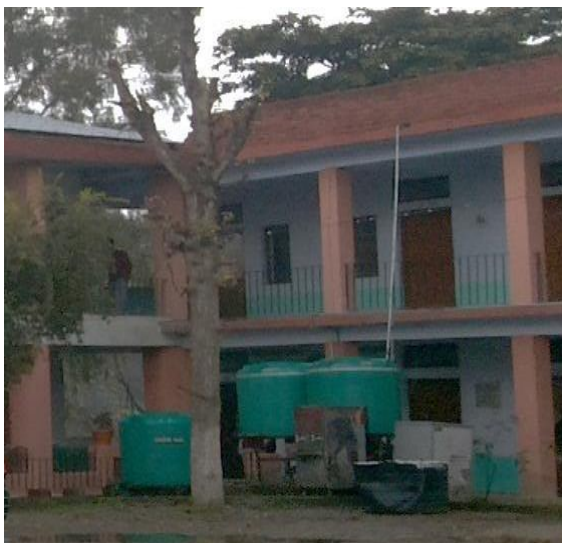
Fig.33 Incorrect setup of rain water harvesting plant (GSSS Nalti)
