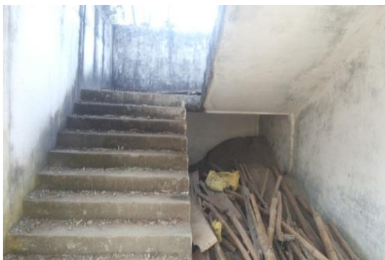
Fig.27 Handrail not installed.(GSSS Bhota)
