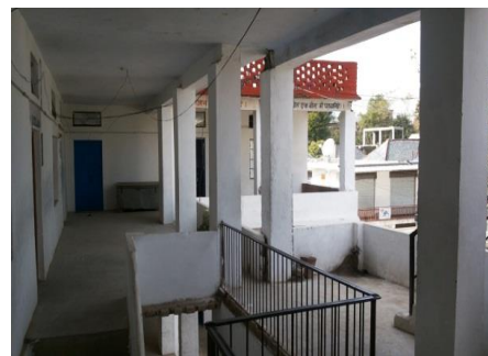
Fig.10 Chaotic construction (GSSS kot)
