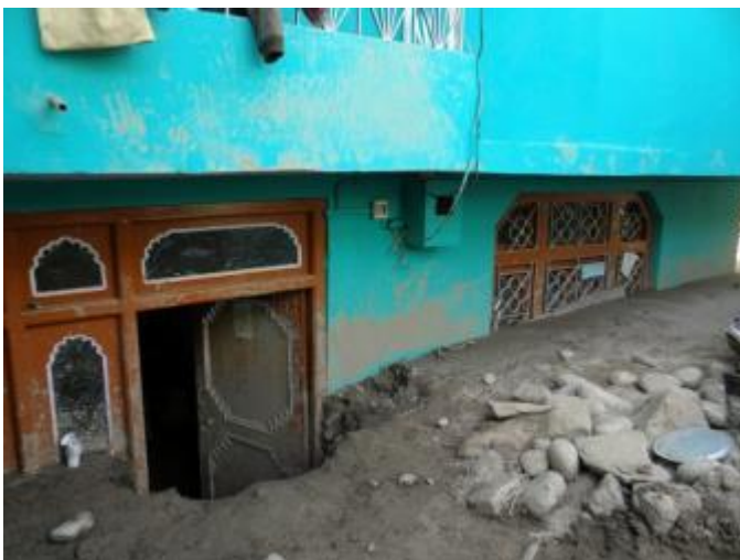
Mud flow covered the houses upto 5-6 feet.
